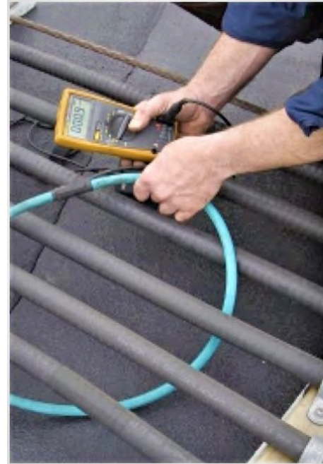
Fig. Ground Fault Location using a portable current sensor connected to a hand held meter.
